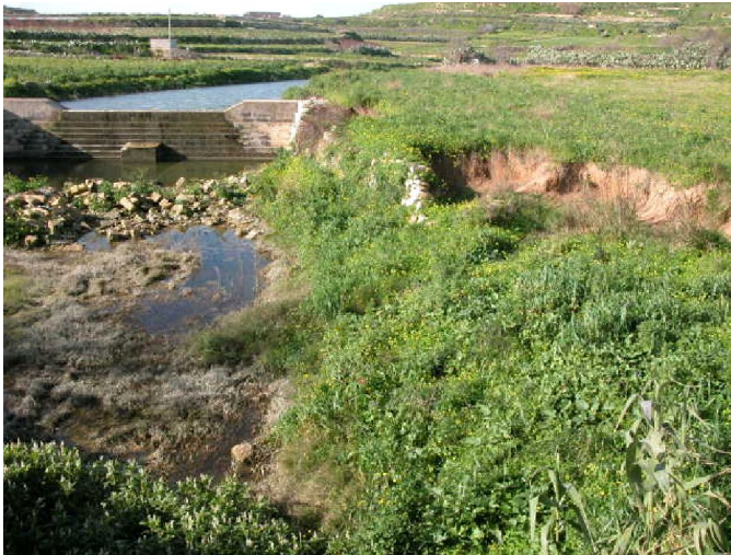
Picture 1. Side walls collapsing into the valley
